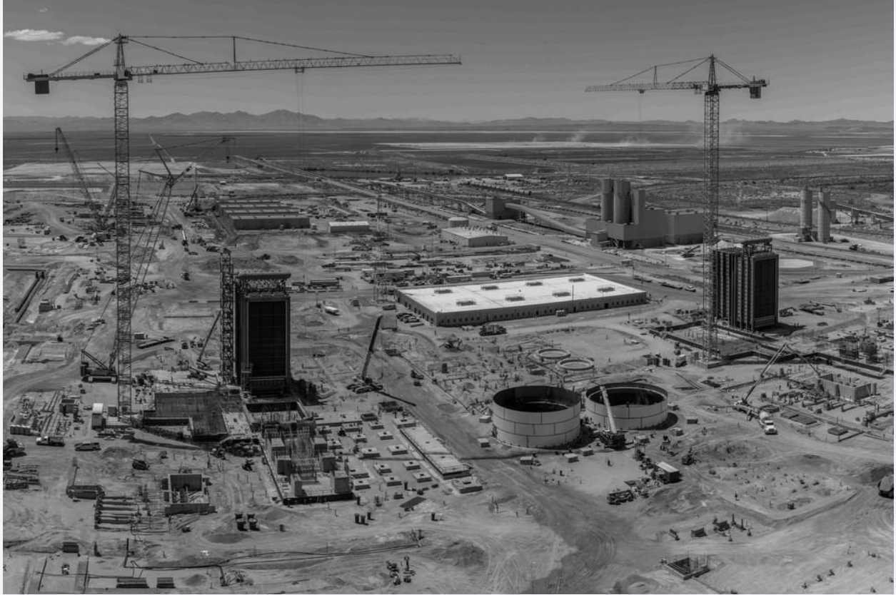
The Mitsubishi Power IPP Renewed site is seen under construction on July 27, 2023, in Delta, Utah. | Business Wire via AP
