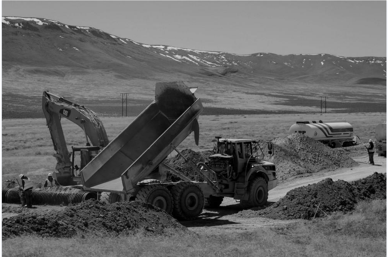
Construction takes place at the Lithium Nevada Corp. Thacker Pass mine site on April 24, 2023, near Orovada, Nevada. | Rick Bowmer/AP
